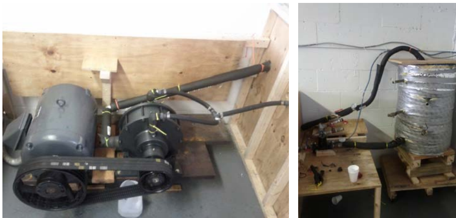
Figure 7: Cavitation heat pump setup to Increase efficiency, elevated water tank and insulated discharge pipes
